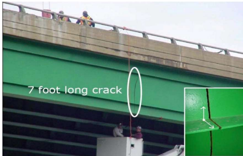
Chajes et al. „Fracture: Field testing of the I-95 bridge.“ In Third Annual Bridge Workshop: Fatigue and Fracture; Center of Innovative Bridge Engineering: Ames, IA, USA, 2004
