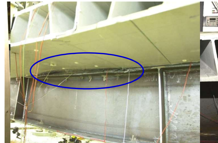
Failure of adhesive bond
