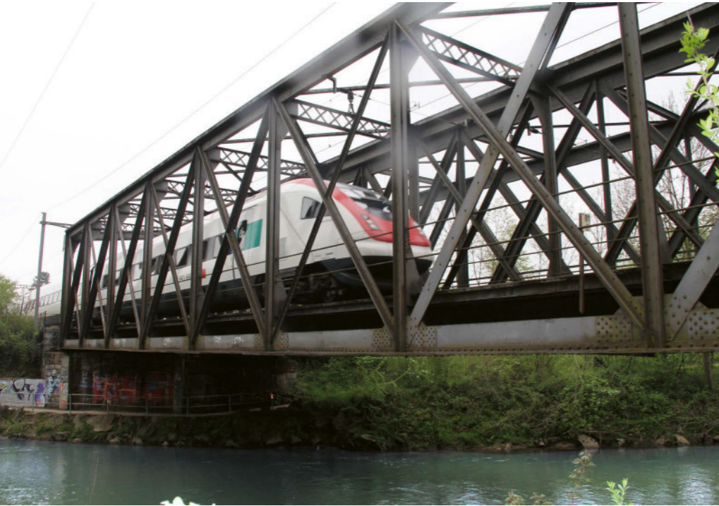
Münchenstein Bridge near Basel was reinforced with CFRP strips back in 2015. Several intercity trains per hour and several goods trains per day roll over the 126-year-old bridge.
